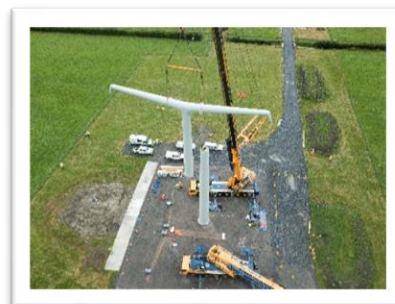
Picture of first T-ylon being constructed in Somerset in September 2021 (taken from National Grid website:
